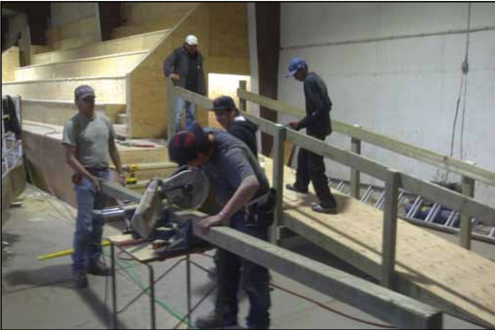
Pre-construction trainees busy during construction phase of work inside the Kainai Agri-plex.
