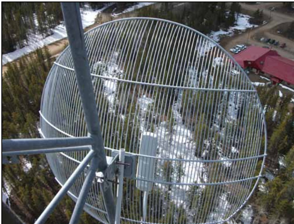
A parabolic antenna overlooks a native community that has integrated the wireless high speed internet system.
