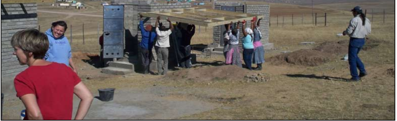
Sanitation units are being assembled in a partnership between Blood Tribe, Canada and South Africa
