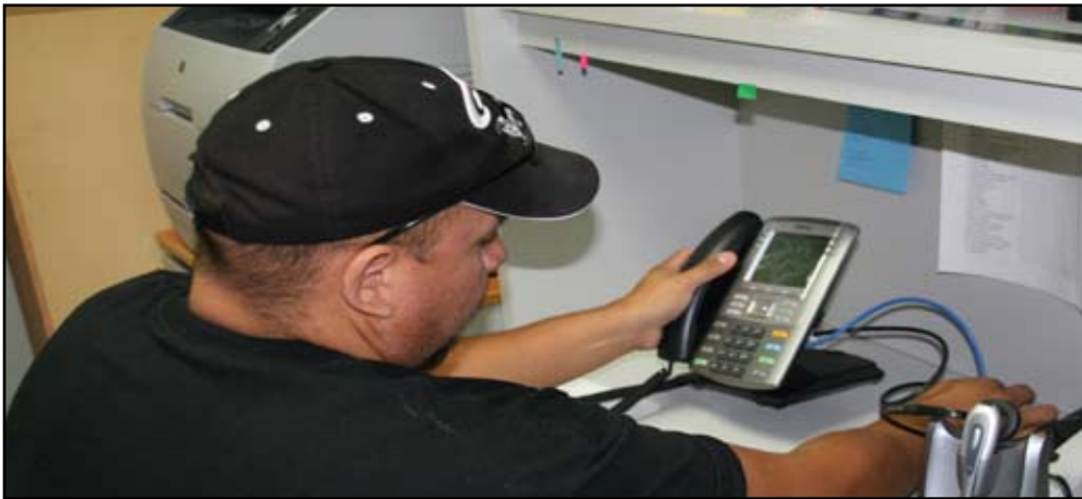
It's been busy for Frank and associates who are installing the new telephone system
